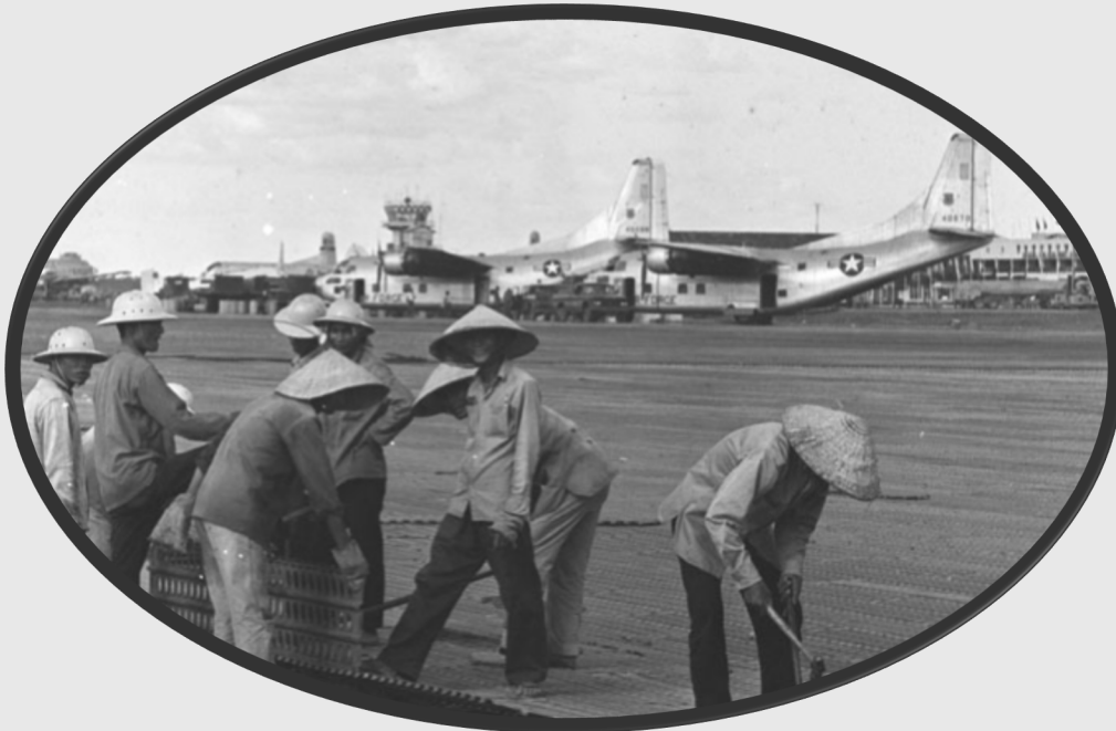
South Vietnamese workers repair the runway at TSN AB, ca. 1970s. (USAF Photo)
